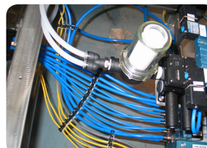
Air line and wire separators
